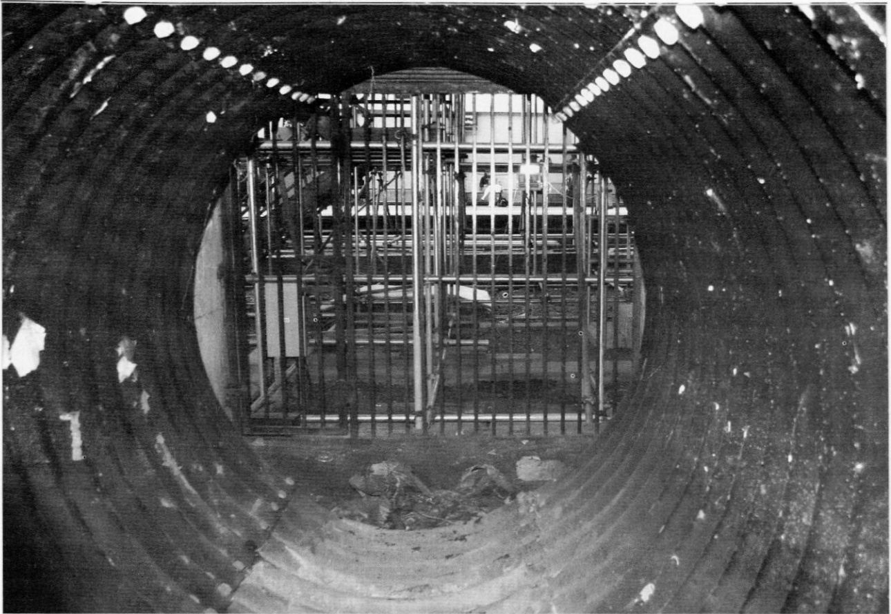
Platform 19 at Waverley Station seen from the tunnel under Waverley Market - Photo by Nick Catford
